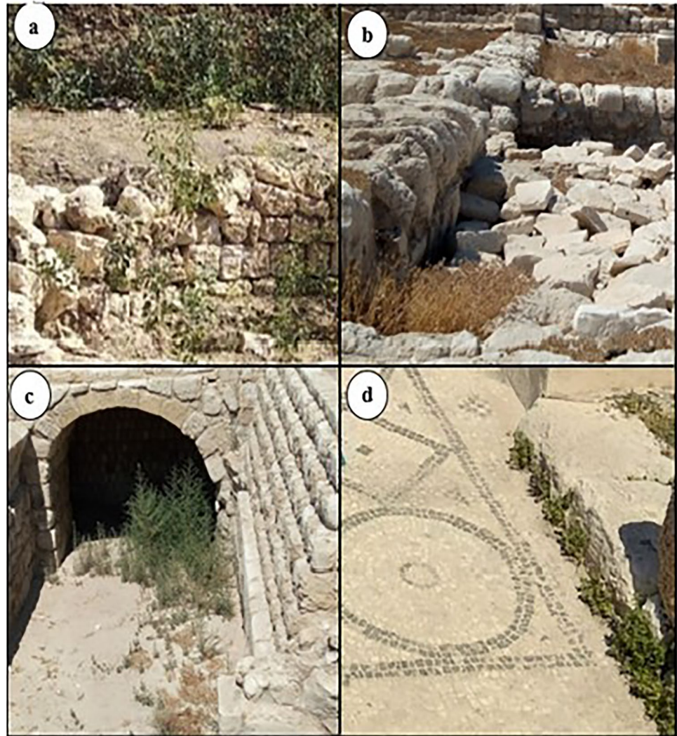
Fig. 1 An example of plant colonization at Kom el Dikka site Alexandria, Egypt ( a and b showing the growth of the plants between stone blocks, c showing plants under the ribbed vault, d showing plants growing on the mosaic (Photos were taken by the co-author Yomna M. Elgohary)
