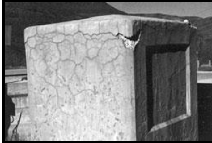
Fig 26: White patches on external walls
