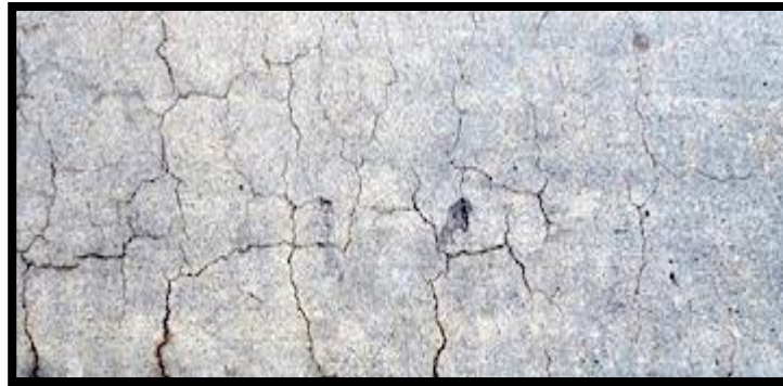
Fig 27: Deterioration of concrete in sea water
