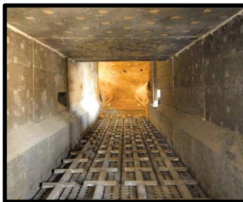
Fig 19: Grate cooler entrance
