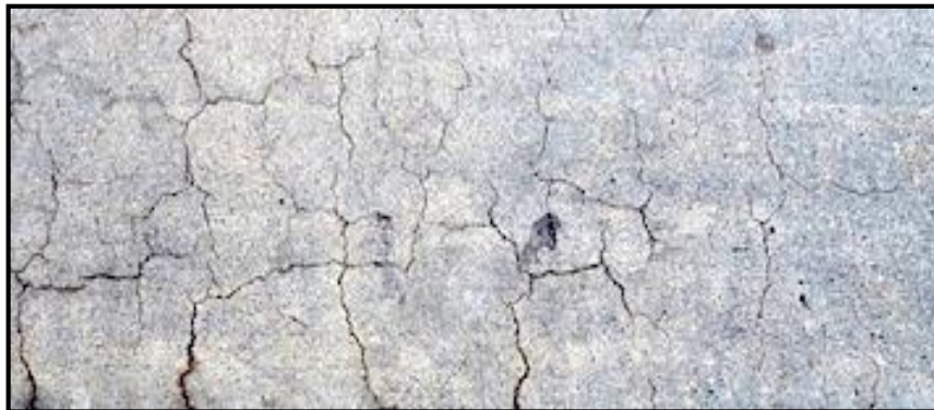
Fig 9.21 Deterioration of concrete in sea water
