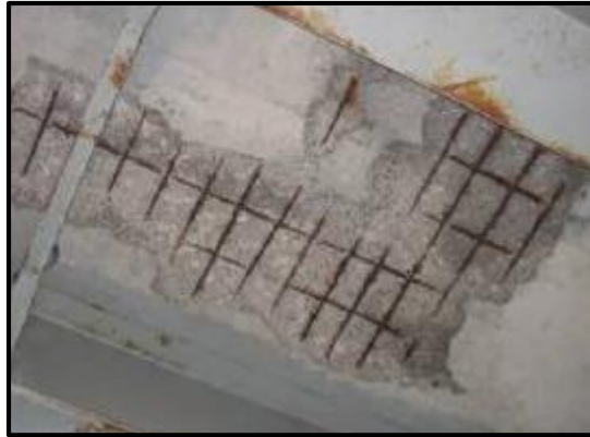
Fig 9.23 Corroded steel bars
