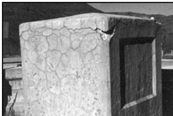
Fig 9.20 White patches on external walls
