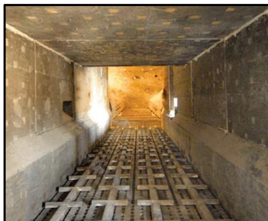
Fig 9.11 Grate cooler entrance
