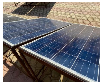
Figure 10: Solar Panel after applying the prepared Nano-coating.
