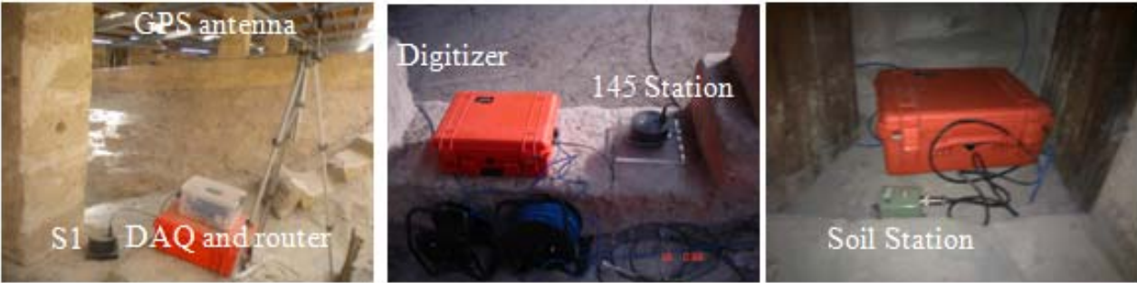
Figure 2. The dynamic system in operation: accelerometer S1, DAQ, router and GPS antenna (left); accelerometer 145-Station and digitizer (middle); and accelerometer Soil-station (right) (Elyamani, 2015).
