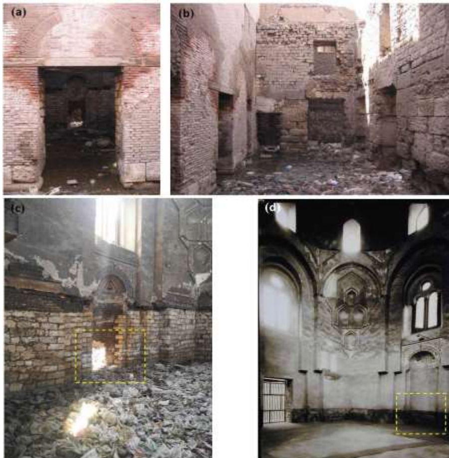
Fig. 1. Current situation of Fatima Khatun Mausoleum: (a) high groundwater penetration by capillarity in masonry walls; (b) local damages and accumulation of groundwater and garbage; (c) garbage dump inside the mausoleum and partial collapse of a wall; (d) historic photo showed no deterioration (source: Creswell collection) [26])
