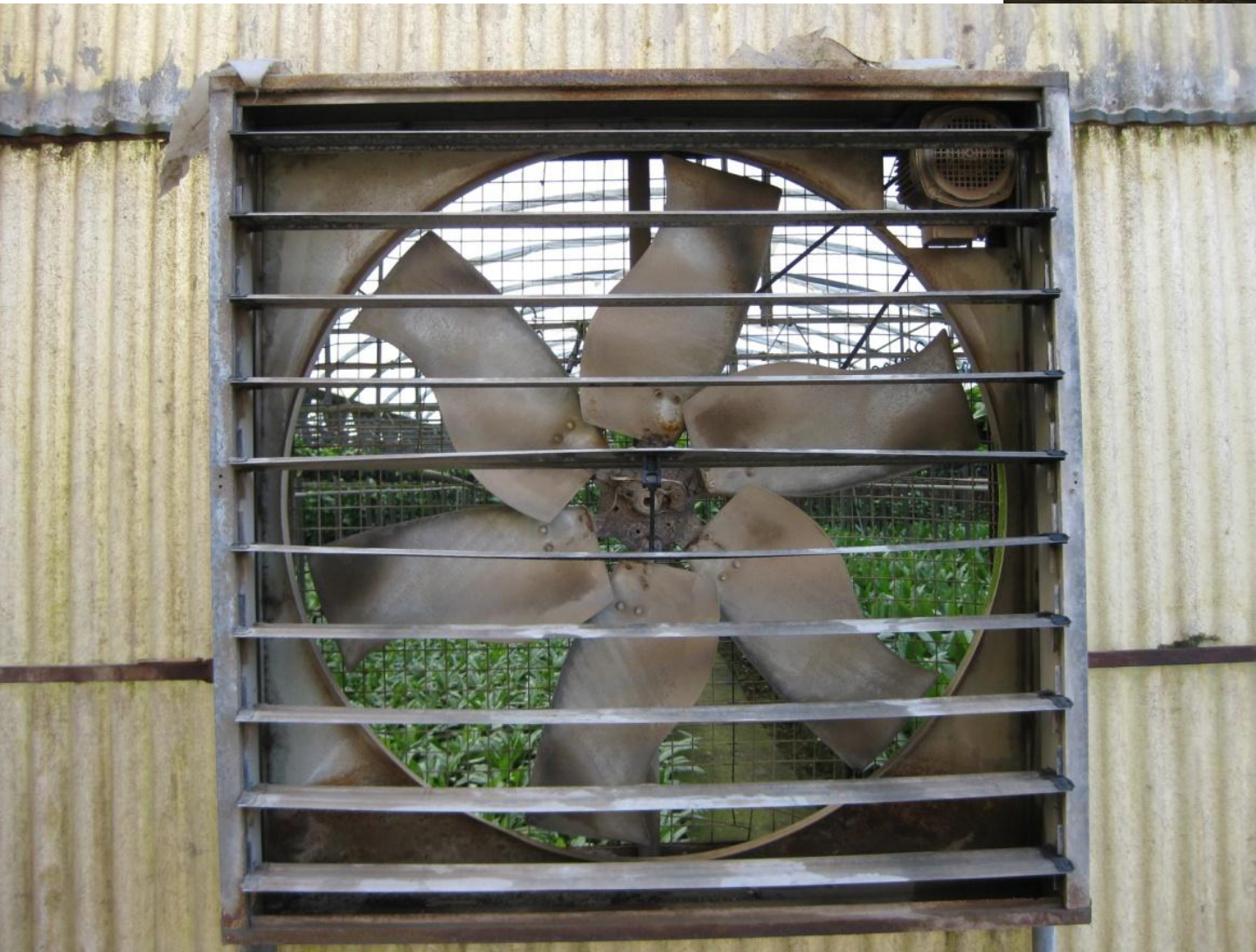
A Vaneaxial Fan in a Greenhouse
