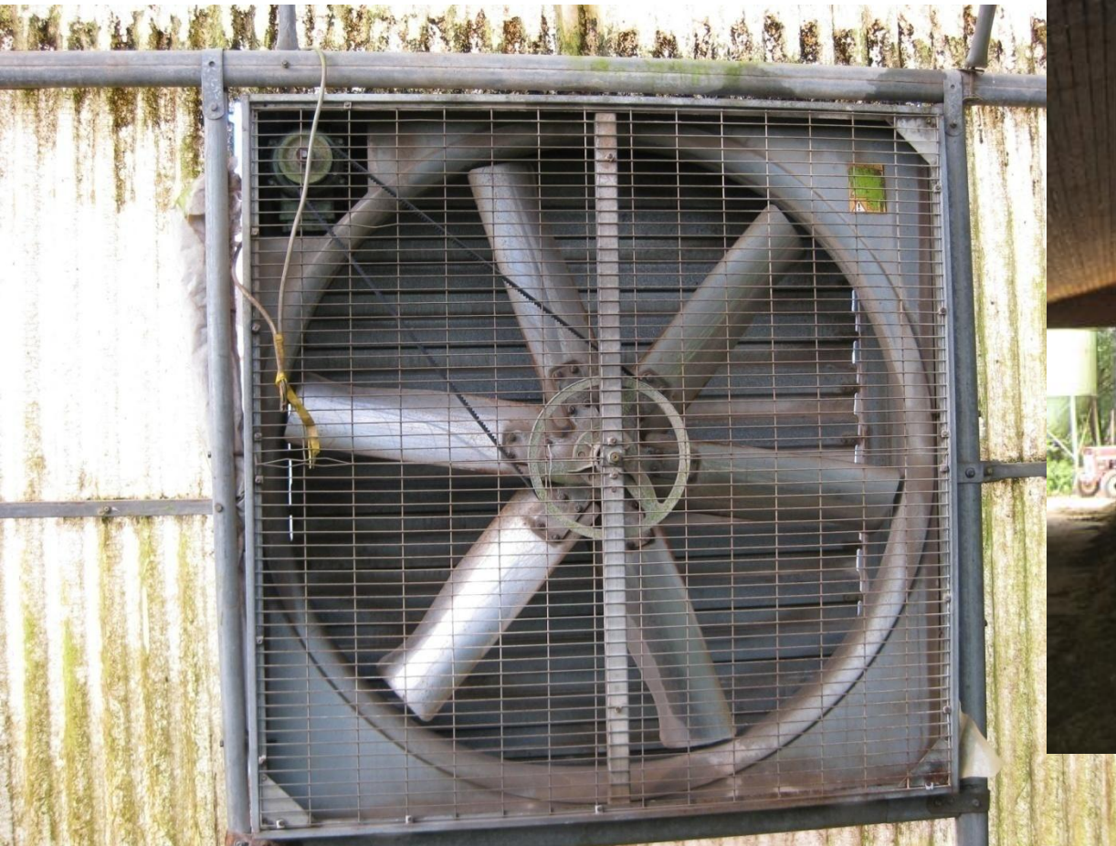
A Tubeaxial Fan in a Greenhouse
