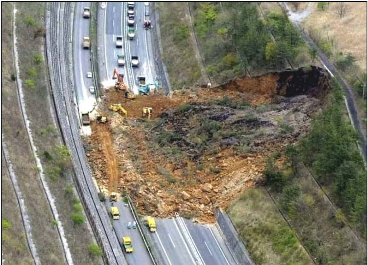
Failure of soil along a curved plane
