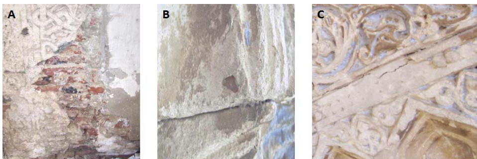
Fig. 4. The application of different treatments: a & b - direct application of stucco mortar and engraving, c - application of two stucco layers on the substrate
