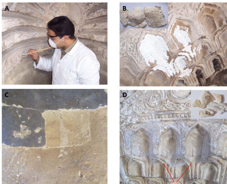
Fig. 5. Photographs during cleaning: a and b - the dusting and application of paper poultice with ethyl alcohol, c and d - the removal of lime layers by mechanical cleaning
