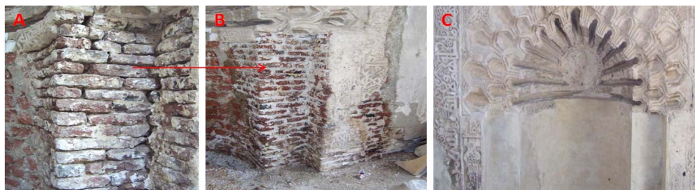
Fig. 10. The stages of removing of Portland cement layer cleaning of brick joints (a), b - the pointing of brick joints, c - the application of porous lime plaster (disposable layer)
